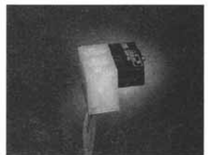
CSF-MH-03-02 on A DB5 Switch
